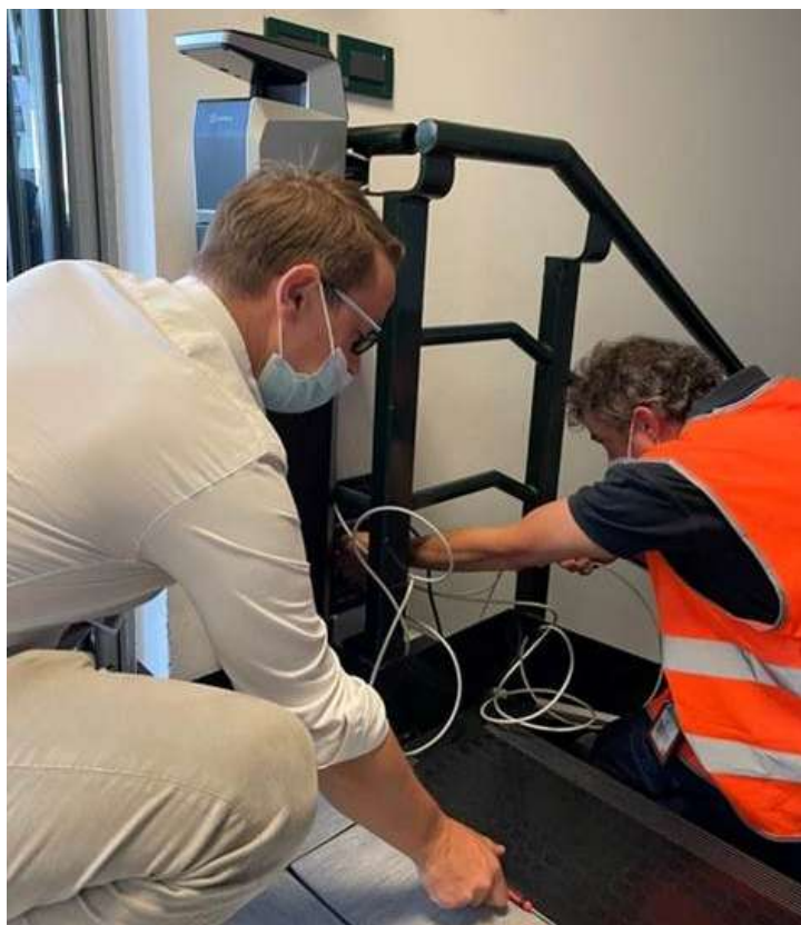
Figure 5: Installation of the Unified Access Control at the AOCC door at Milan Malpensa Airport premises
